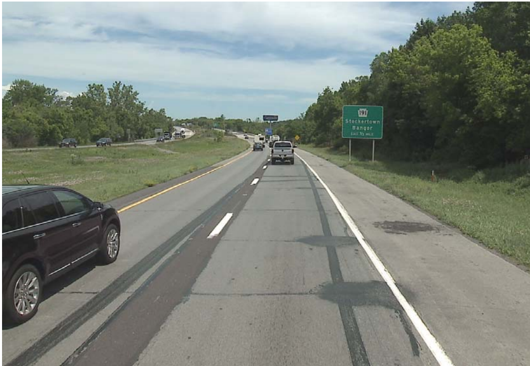
Northbound – County Repairs Longitudinal Joint Patch, Transverse Cracks, and Transverse Joint Spray Patching
