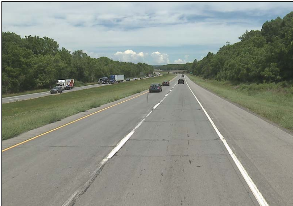
Northbound Travel Lane Typical Pavement Condition
