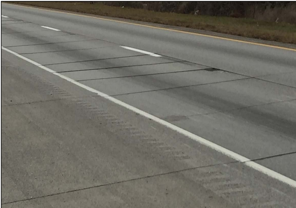
Eastbound Travel Lane – Segment 0700 Typical Pavement Condition (Bituminous Patching Area)
