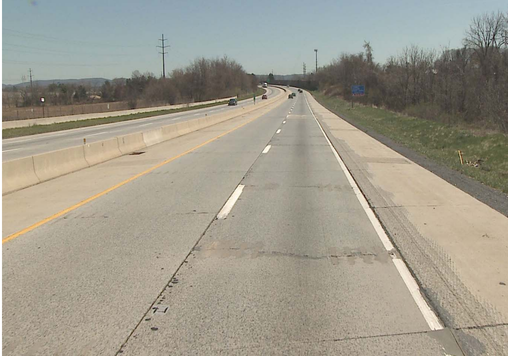
Eastbound Travel Lane – Segment 0524 (Lehigh County) Concrete Patching Pavement Condition
