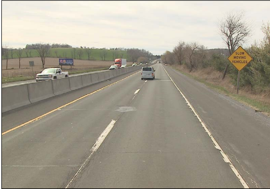
Westbound Passing Lane - Segment 0475 (Lehigh County) Typical Pavement Condition
